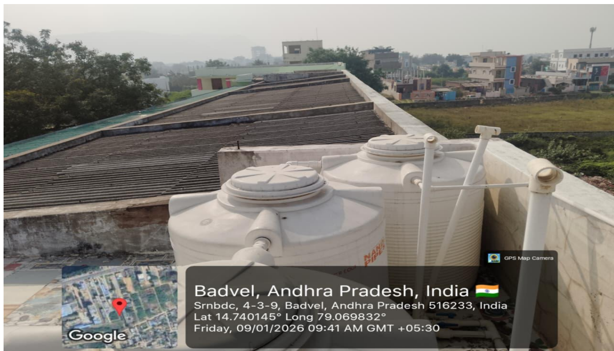
Figure: 1 RO System Control Panel with Storage Tanks at SRNBDC Campus-2
