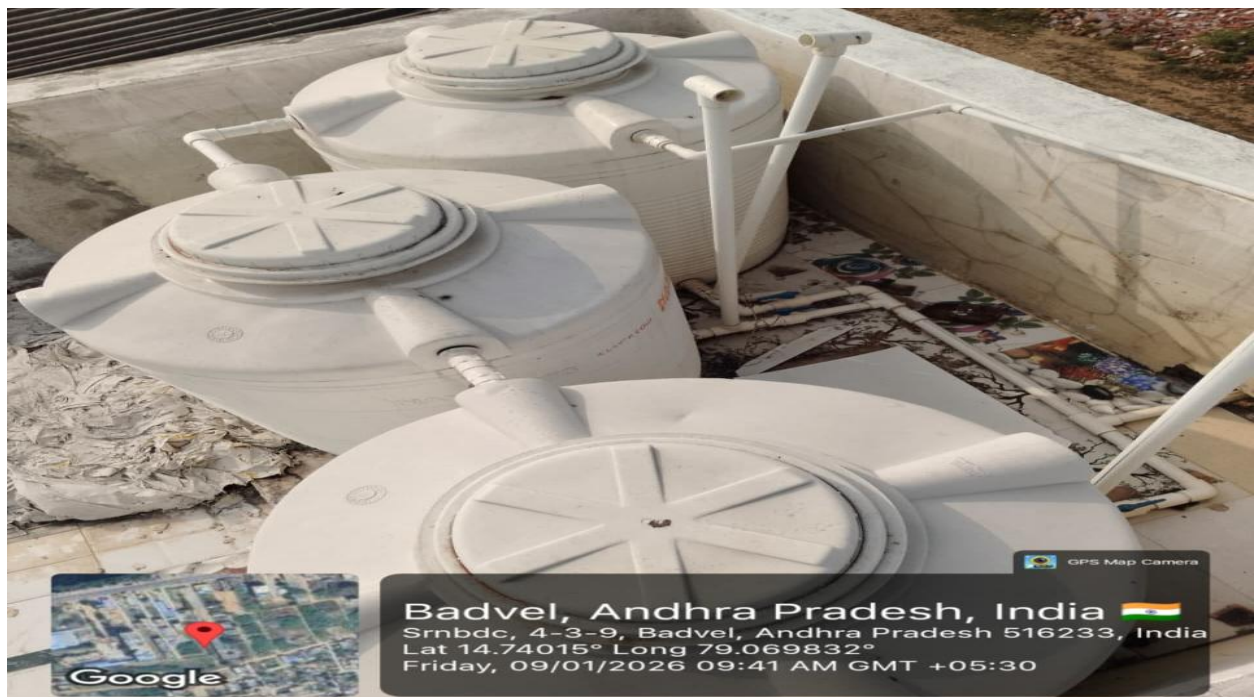
Figure-2 RO Plant generated Waste water can be stored in Tanker
