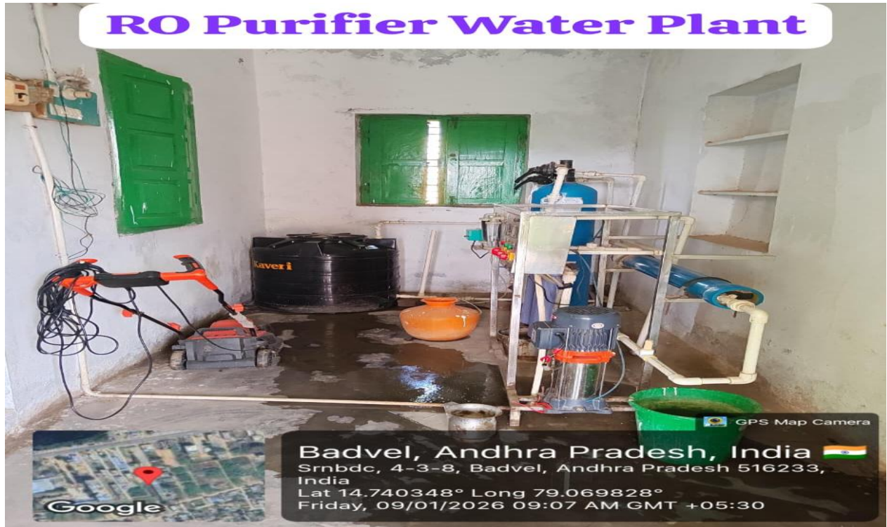
Figure-1 RO Plant generated Waste water can be stored in Tanker
