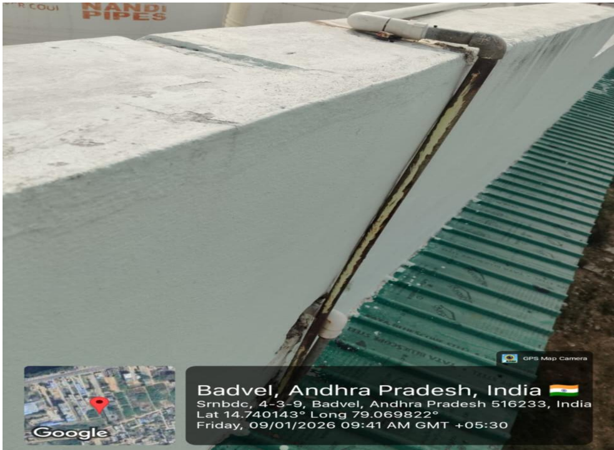
Figure-5 Waste Water pipelines from RO System on wall f the building-2
