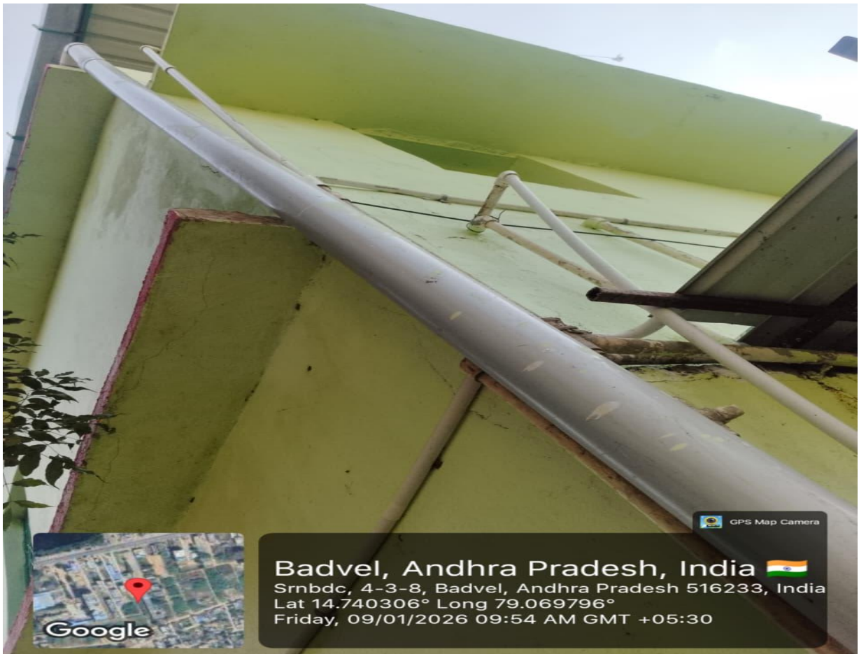
Figure-4 Waste Water pipeline from RO System on terrace of Building
