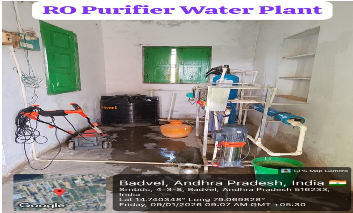
Figure: 1 RO System Control Panel with Storage Tanks at SRNBDC Campus-1
