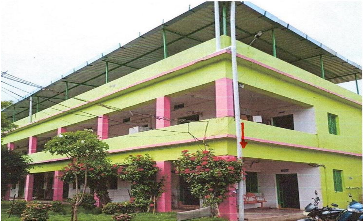
Figure-3 Waste Water pipeline from RO System on terrace of Building
